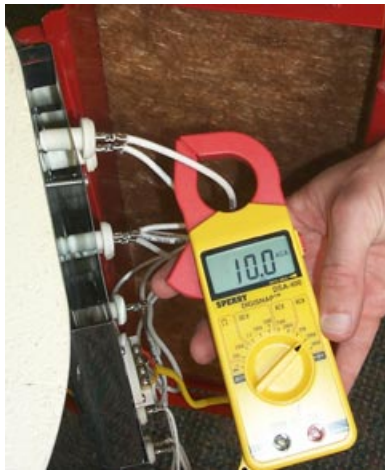
Testing Amperage at Feeder Wires
