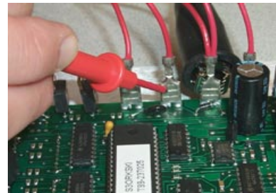
Measuring Controller Voltage
